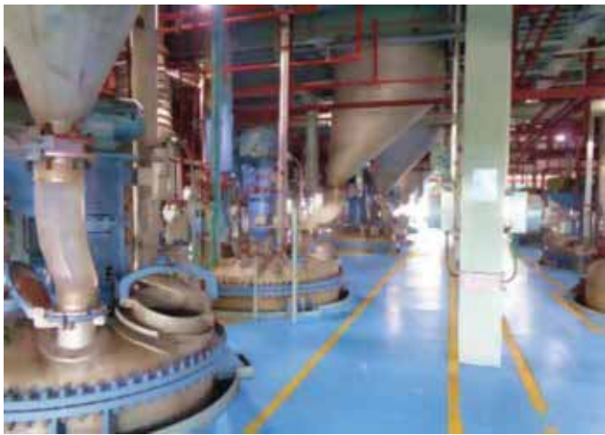
Resin Manufacturing setup with modernised safety systems commissioned at Jejuri
