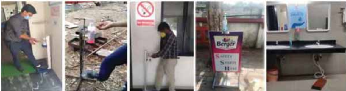
In-house fabricated foot operated sanitizer dispenser, wash basins & motion sensor taps
