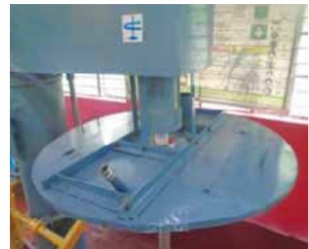
Open Mouth vortex stirrers are converted to closed mouth arrangement to minimize VOC emissions and lead towards safer operations
