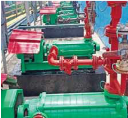
Conventional Pump seals are replaced with Mechanical seals which ensures no leakage and spillage free dykes.
