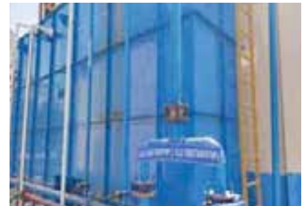
Efficient domestic water treatment through STP (Sewage Treatment Plant) at VVN
