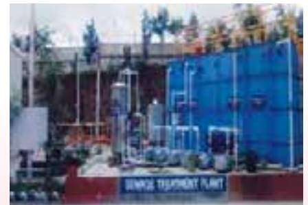
Compact and Modern Sewage Treatment Plant at Jejuri Plant
