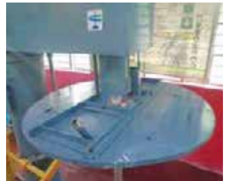
Open Mouth vortex stirrers are converted to closed mouth arrangement to minimize VOC emissions and lead towards safer operations
